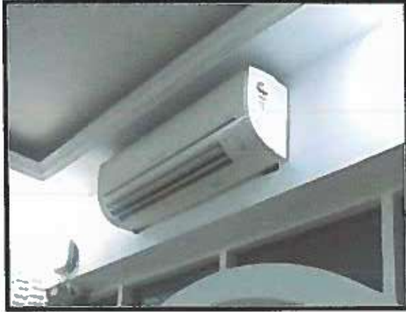
Air Conditioners Installed in Lab
