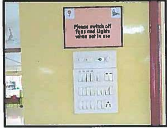
Signages near switch boards
